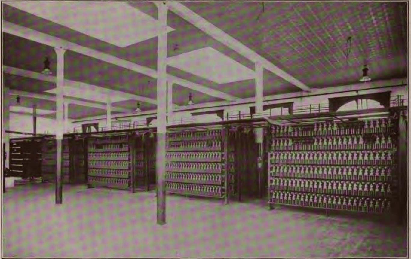
CENTRAL AUTOMATIC EXCHANGE, GRAND RAPIDS, MICHIGAN, 6,000 LINE FULL AUTOMATIC.
